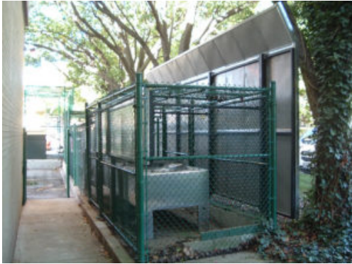
This acoustical barrier helps mitigate the noise disturbance of a building's air conditioner units.
